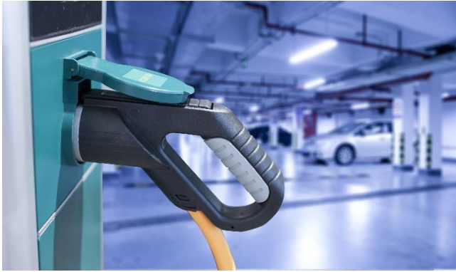
Figure 1. Charging station for e-mobility in an underground parking garage.
